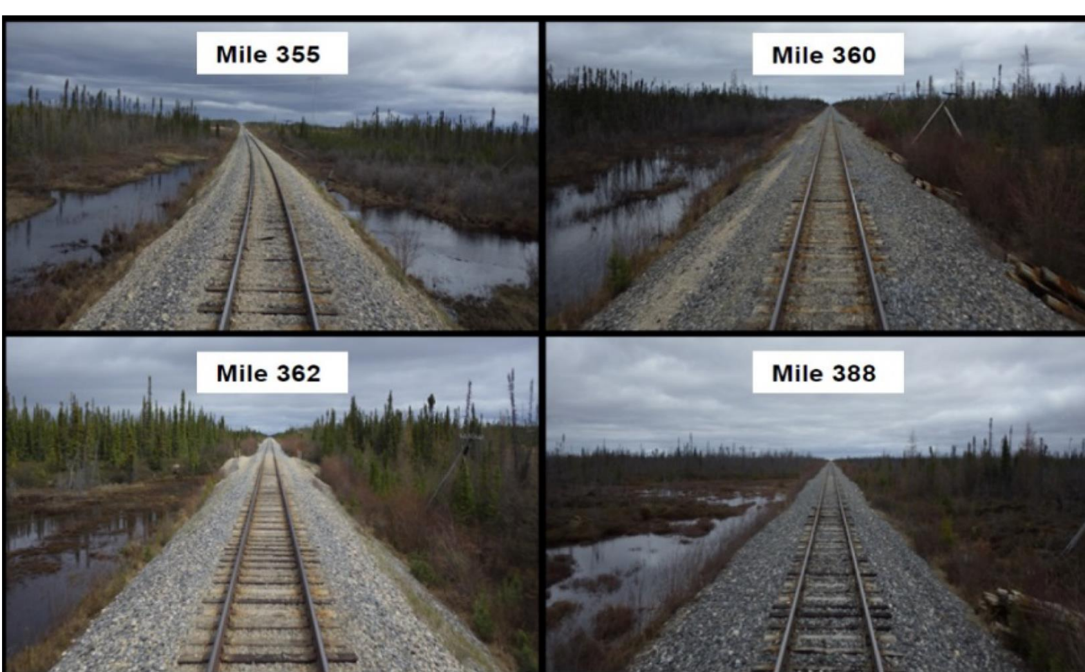
Figure 4: Drainage condition along HBR (Oommen et al. 2017).
