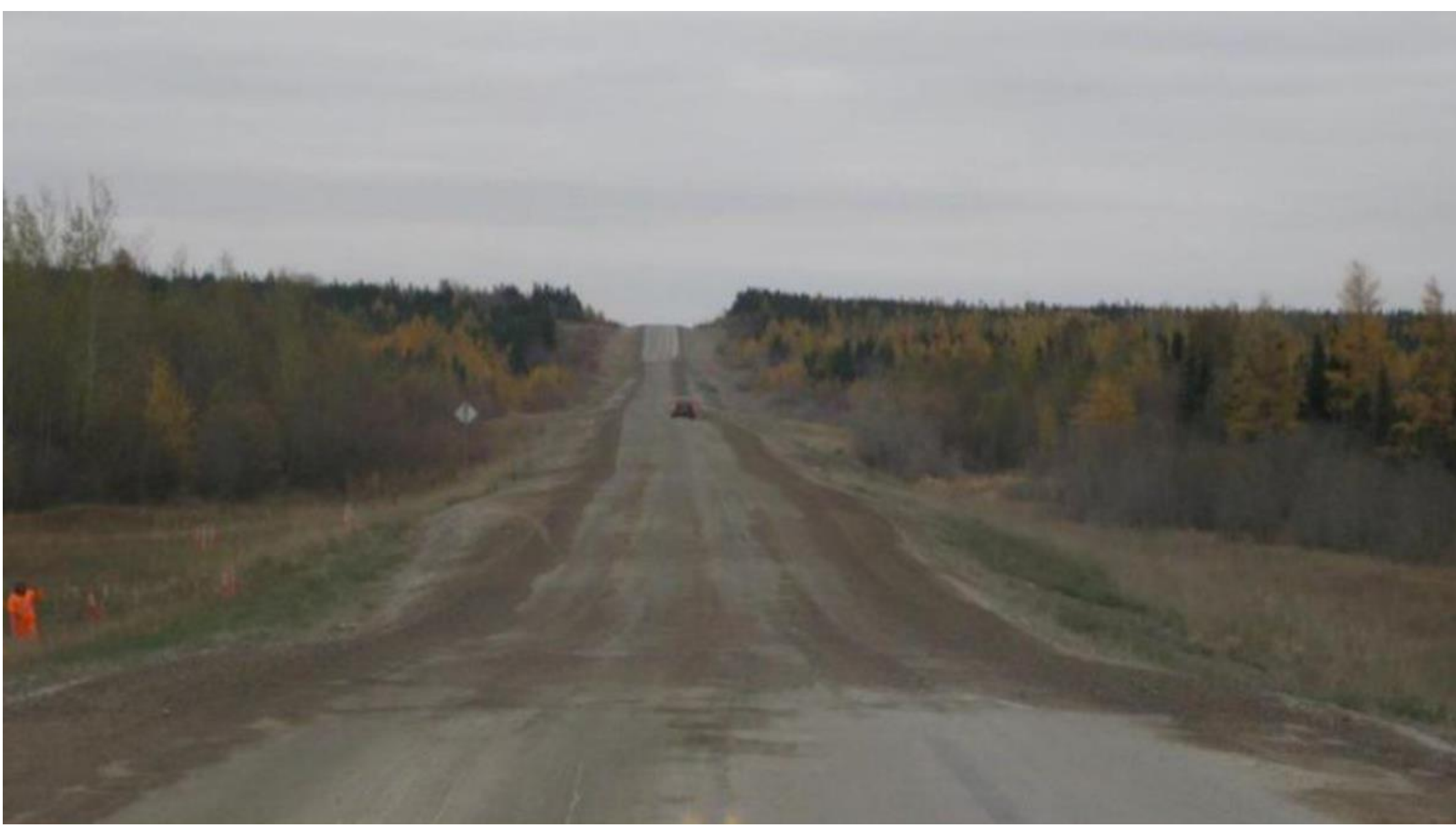
Figure 3: Settlement of the road due to the permafrost degradation (Batenipour et al. 2014).
